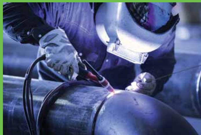
A typical application of walking the cup in the GTAW/TIG welding of piping.
